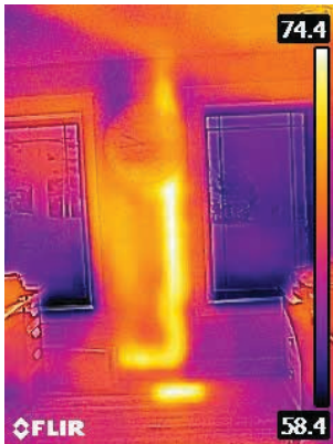
Warm Drain Pipe in Wall
